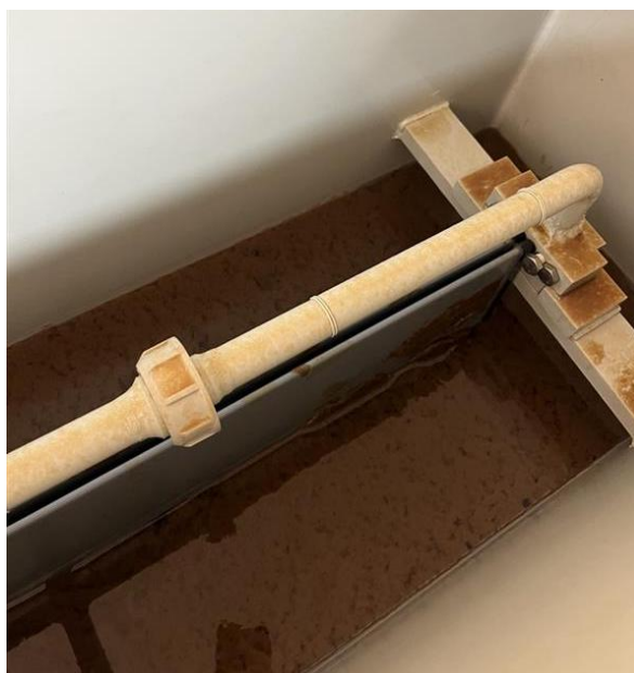
Figure 11. Sludge in the bottom of the membrane tank.
