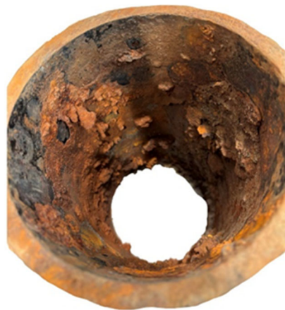
Figure 1: Cast iron pipe that was installed in 1910 in Norrvatten's DWDS.
